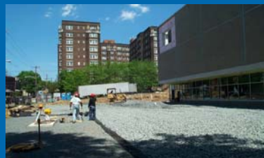
Recharge Bed under Porous Pavement Play Yard
